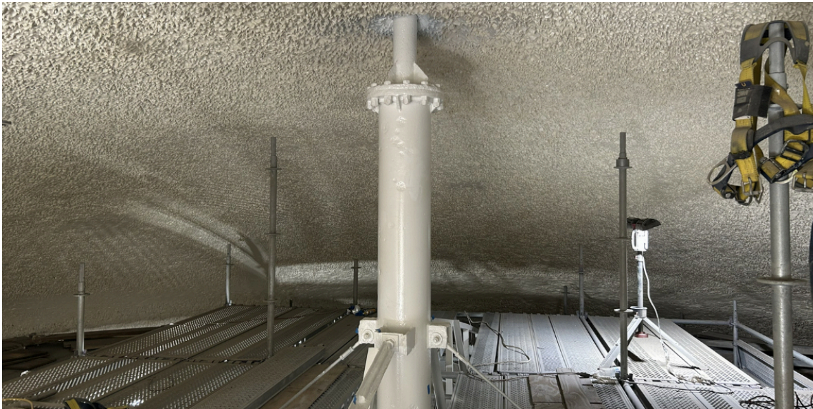
Pictured above, is the North Vacuator located at the Water Resource Recovery Facility.
