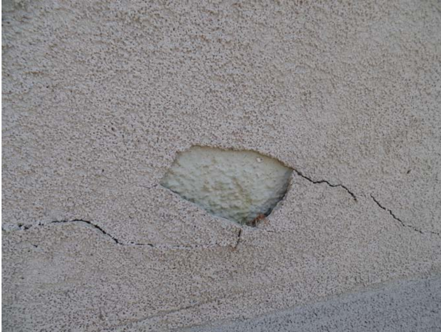
Figure 22. View of older stucco cladding still extant under newer application of stucco to 24765 Hesperian Boulevard (Garavaglia Architecture, Inc.)
