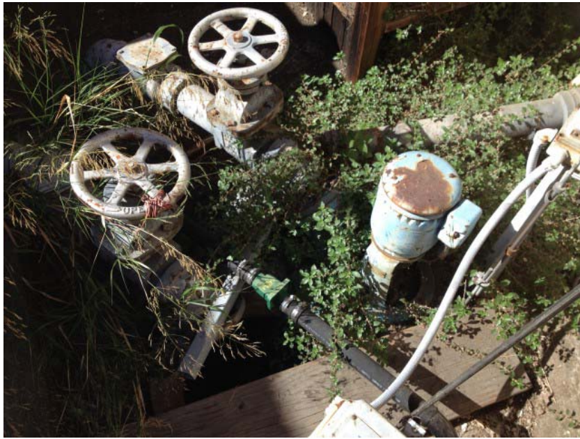
Photo 1. View of waste water outfall located in interior courtyard area. Photograph taken on October 21, 2014.
