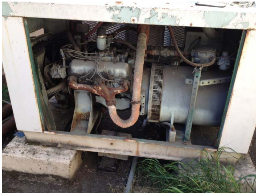
Photo 2. View of internal combustion powered generator located in interior courtyard of subject property. Photograph taken on October 21, 2014.
