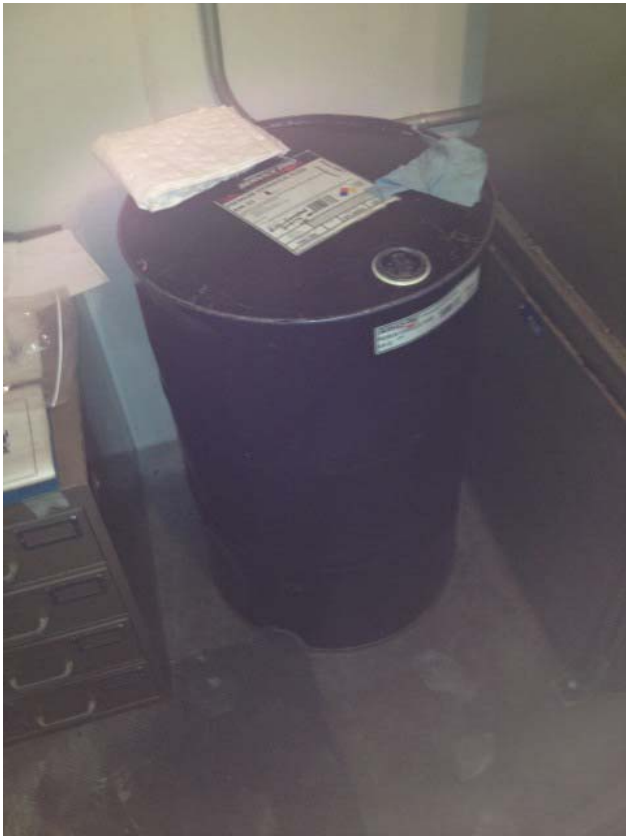
Photo 1. View of hydraulic oil stored in basement-level elevator machine room. Photograph taken on October 21, 2014.
