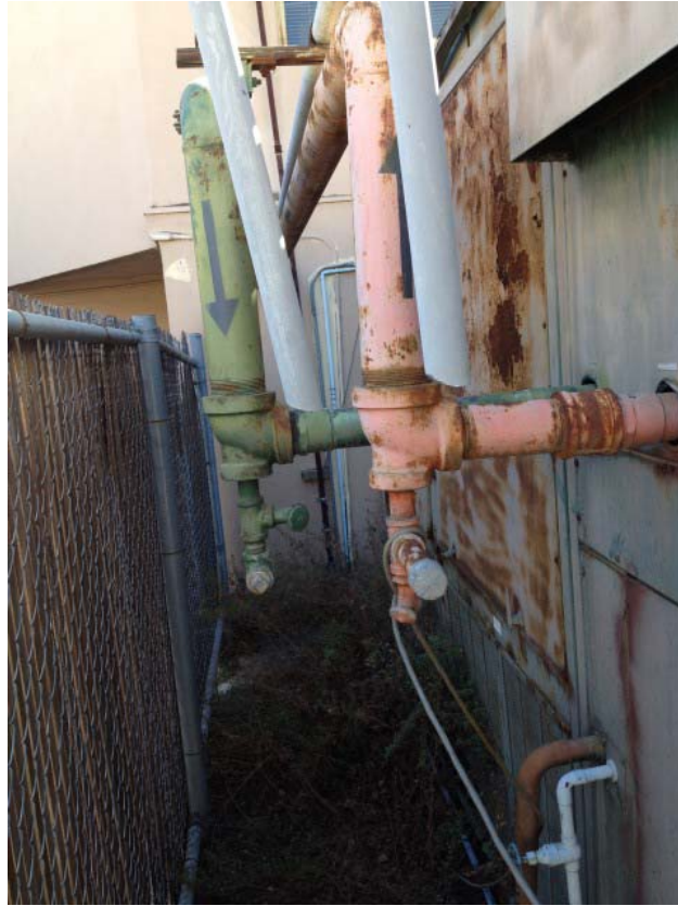
Photo 1. View of natural gas-powered boiler located in backyard of 1013 McKeever Avenue. Photograph taken on October 21, 2014.
