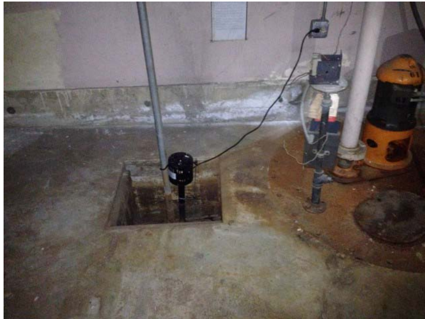
Photo 2. View of sump and associated pump in basement. Photograph taken on October 21, 2014.
