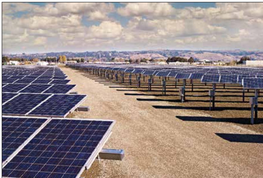
FIGURE 2 - One Megawatt Solar Array
