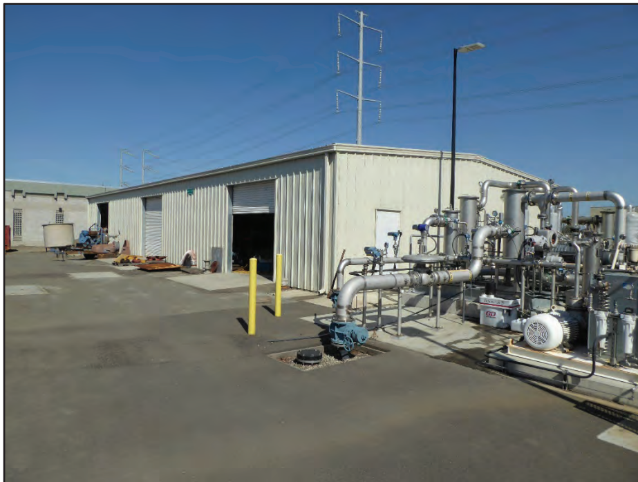
Photograph 41. Building 37 (Warehouse, center) with Structure 36 (Gas Conditioning Area, foreground right) and Building 44 (Solids Thickening Building, background left); camera facing northwest, April 21, 2017.
