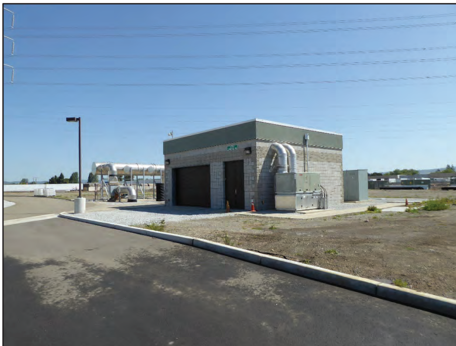
Photograph 45. Structure 42 (East Substation); camera facing northeast, April 21, 2017.
