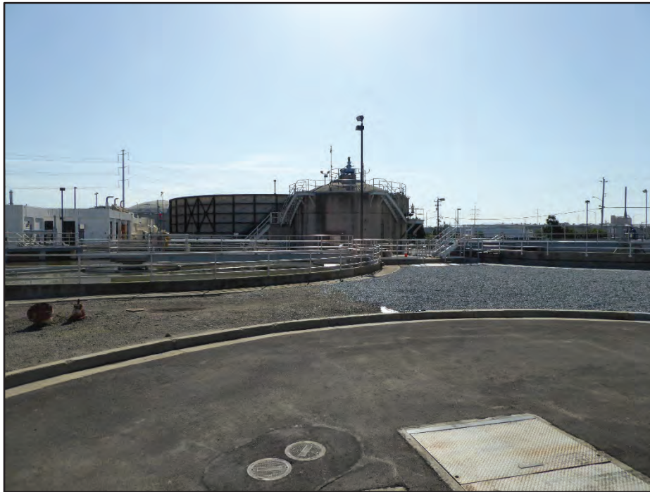
Photograph 6. Structure 6 (South Vacuator, center), with Structure 4 (Northwest Primary Clarifier, left), Structure 5 (Southwest Primary Clarifier, right), and Structure 1 (West Trickling Filter, background); camera facing east, April 21, 2017.
