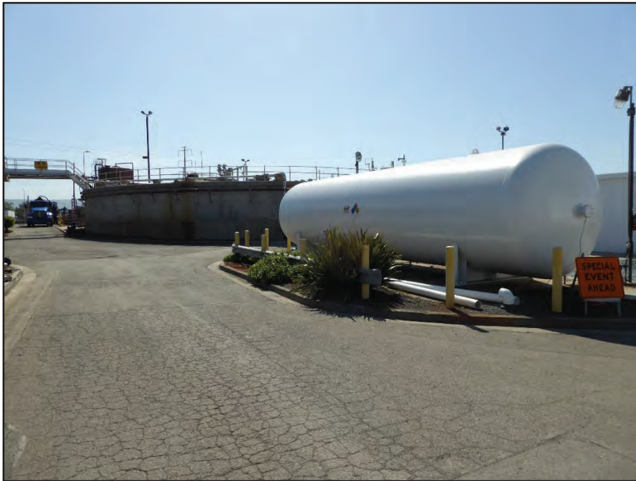
Photograph 30. Structure 26 (Gas Meter Installation) with Structure 12 (Digester No. 2, background); camera facing southeast, April 21, 2017.
