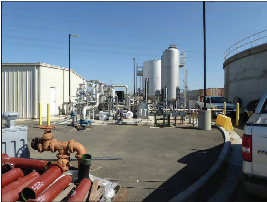
Photograph 40. Structure 36 (Gas Conditioning Area) with Structure 23 (Digester No. 1, right) and Building 37 (Warehouse, left); camera facing north, April 21, 2017.
