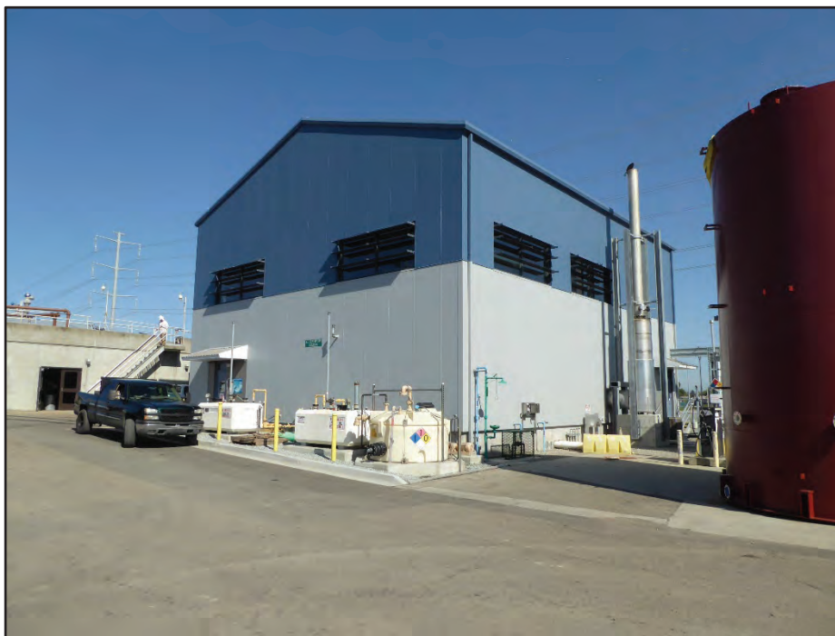
Photograph 42. Building 38 (Cogeneration Building) with Structure 24 (Waste Gas Burner, right); camera facing northwest, April 21, 2017.
