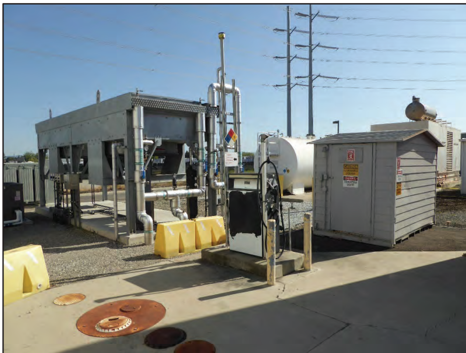
Photograph 27. Structure 24 (Waste Gas Burner); camera facing northeast, April 21, 2017.
