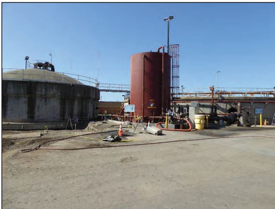
Photograph 22. Structure 18 (FOG Receiving Station, center), with Structure 12 (Digester No. 2, right) and Structure 13 (North Vacuator, left); camera facing south, April 21, 2017.
