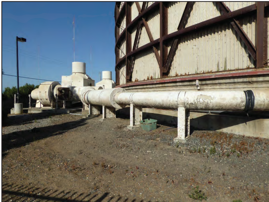
Photograph 3. Detail view of Structure 1 south-side pumping equipment; camera facing west, April 21, 2017.
