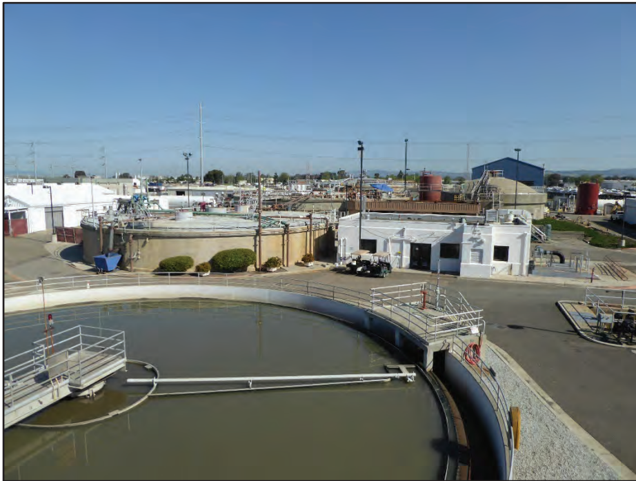
Photograph 8. Building 8 (Site Waste Pump Station & Control House, center right), with Structure 7 (Digester No. 3, center left) and Structure 4 (Northwest Primary Clarifier, foreground); camera facing northwest, April 21, 2017.
