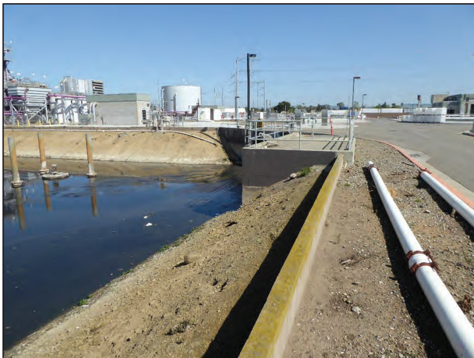
Photograph 11. Detail view of concrete platform at northeast corner of Structure 10; camera facing north, April 21, 2017.
