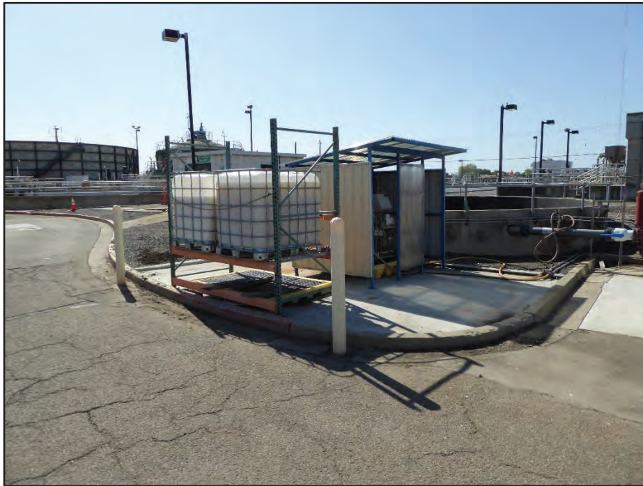
Photograph 52. Structure 50 (No. 3 Water System, center) with Structure 14 (Sludge Conditioning Tank, right) and Structure 1 (West Trickling Filter, background left); camera facing southeast, April 21, 2017.
