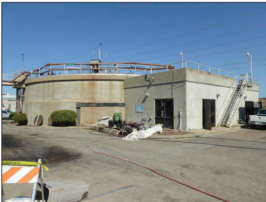
Photograph 26. Structure 23 (Digester No. 3, left) with Building 28 (Mixing and Heating Building, right); camera facing northwest, April 21, 2017.
