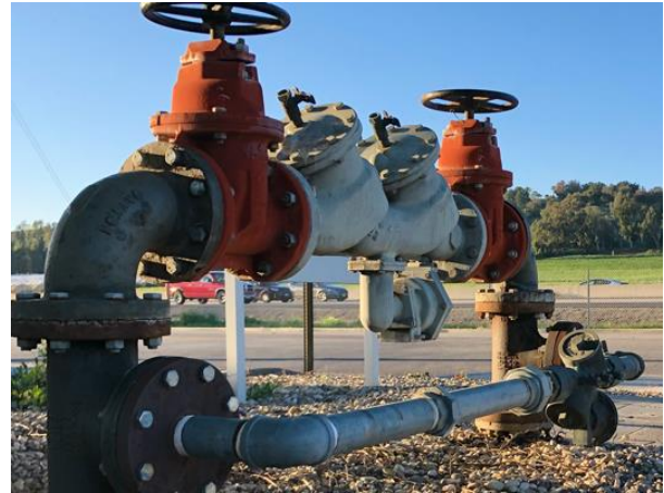
Example of a Backflow Prevention Assembly (USC Foundation for Cross-Connection Control and Hydraulic Research)
