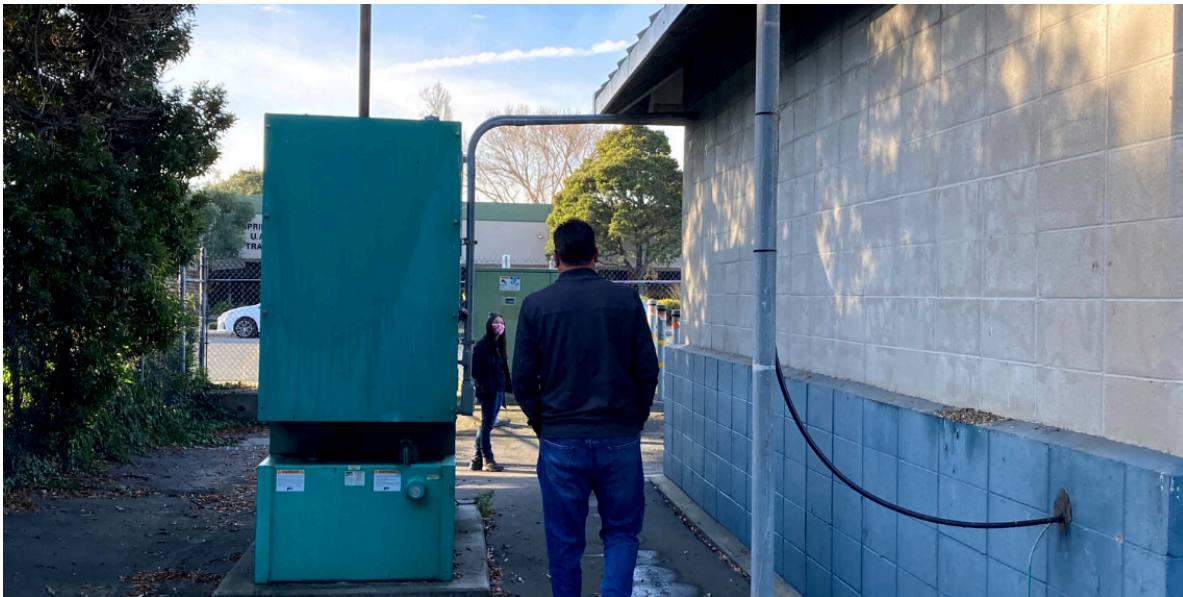
Pictured above, staff inspect the exterior of the Marathon Lift Station, located on Cabot Blvd. Lift stations move wastewater through segments of the City's sewer infrastructure which rise in elevation, and therefore cannot rely on gravity.
