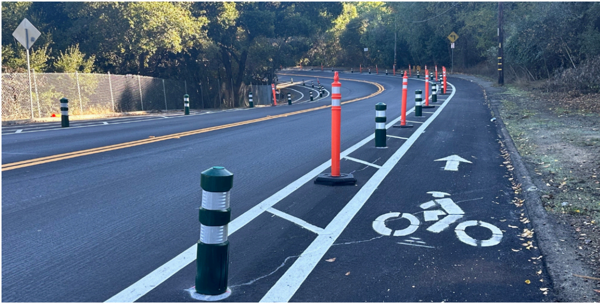
| Pictured above are vertical poles installed as part of the traffic calming pilot program on Campus Drive.
