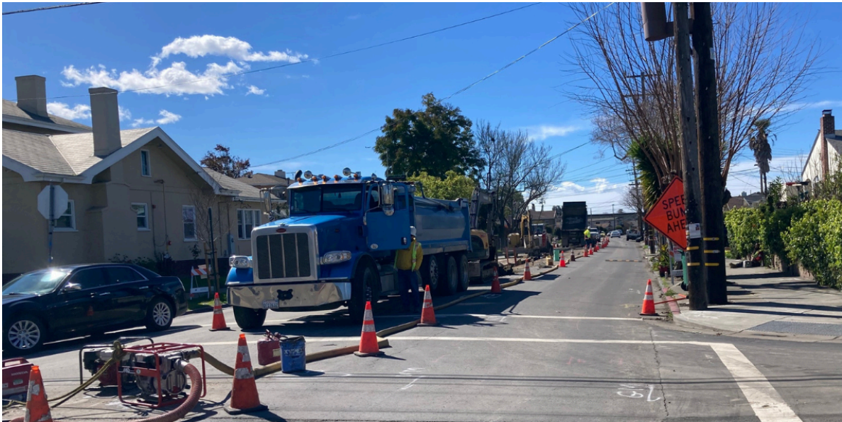
Pictured above: Excavation and installation of new Sanitary Sewer main at Sunset Boulevard and Montgomery Avenue. Temporary Traffic Control and a sewer bypass have been set up as part of the construction operations.
