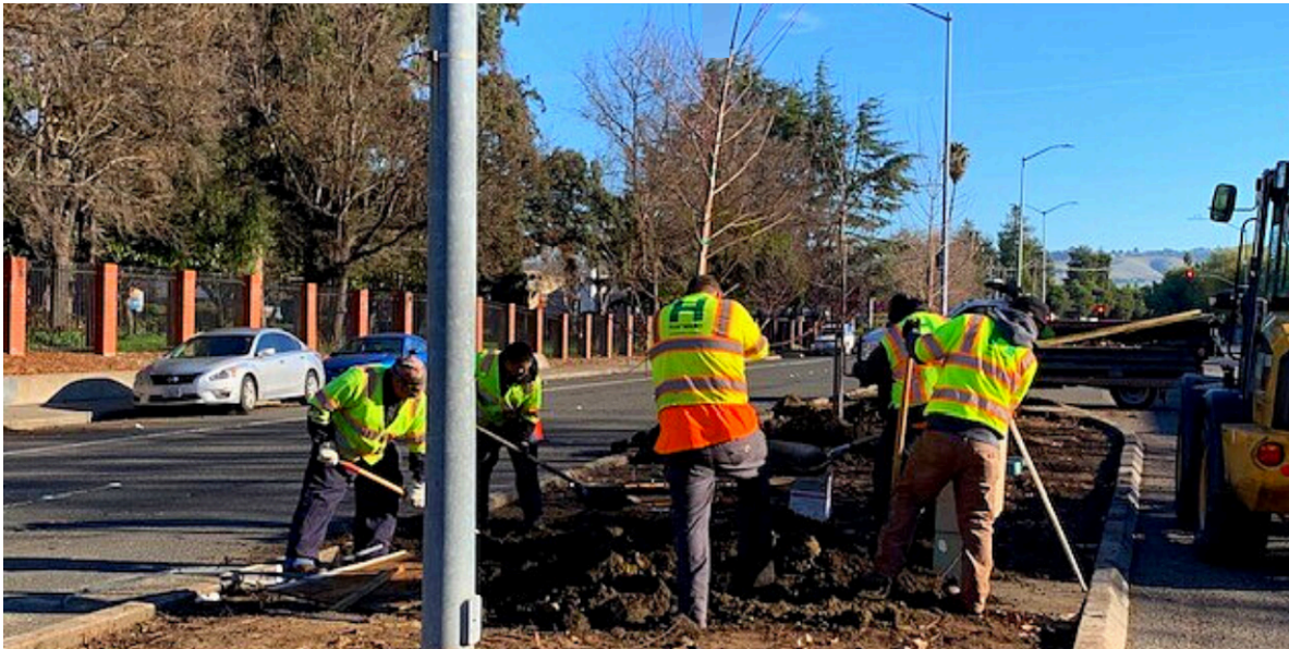
Pictured above, crews work to beautify the Tennyson Corridor median. Similar improvements recently began along the Jackson Corridor in FY23.
