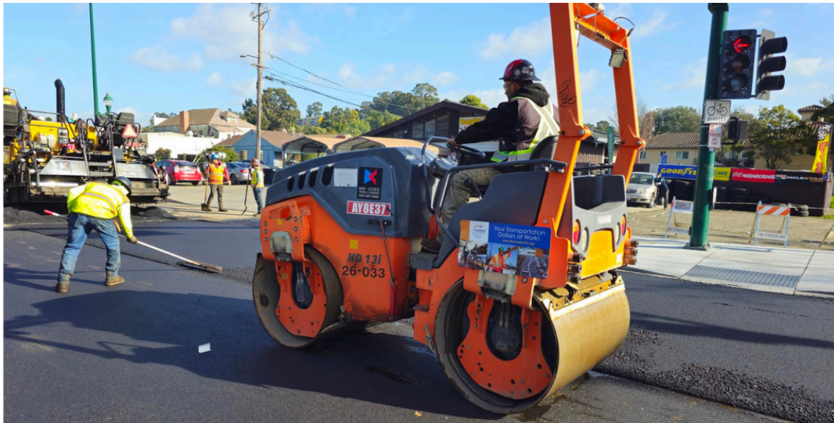
| Pictured above: Crews working to repave intersection of Watkins Street and D Street.
